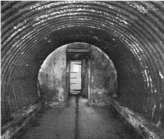
An auxiliary unit's hide in the grounds of Coleshill House that was used for training. Photo: Nick Catford
